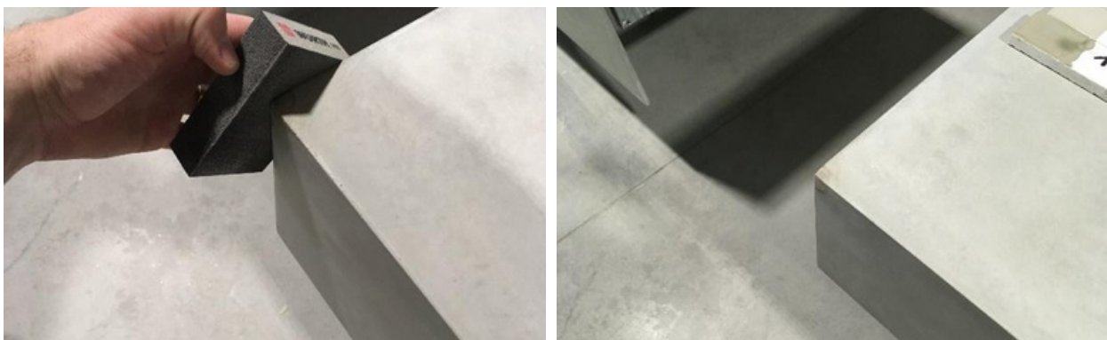
Photo: Example of additional sanding of the repaired area and its final appearance
